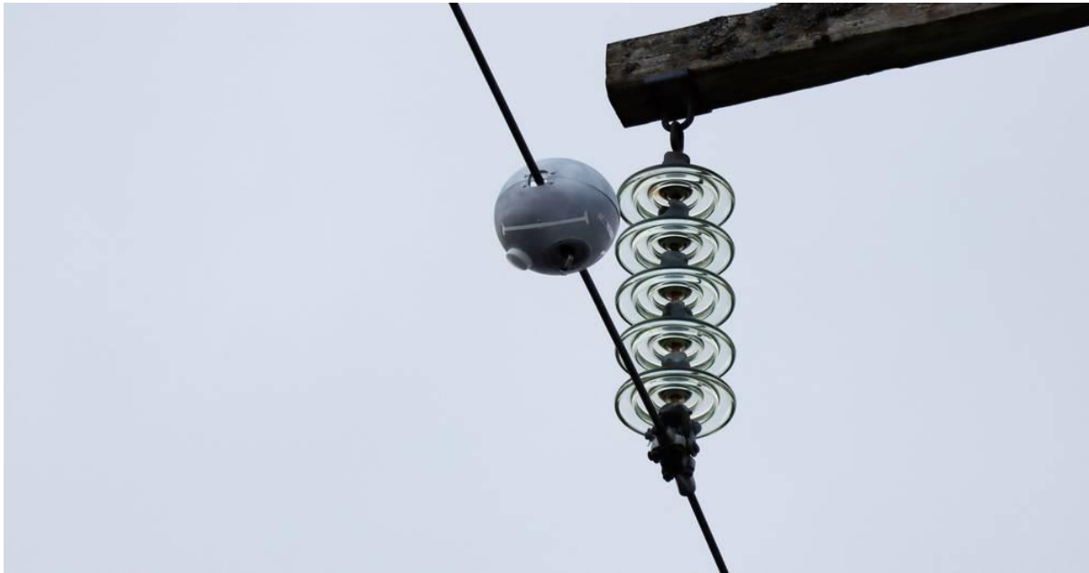
Figure 15: IoT sensor installed on the powerline
