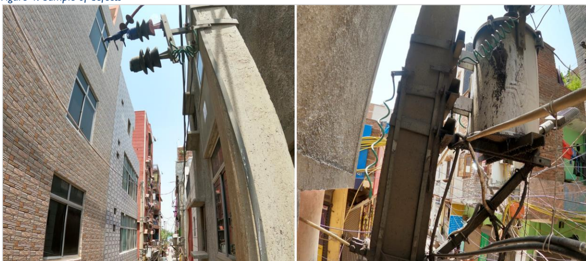
Figure 4: Sample of defects
